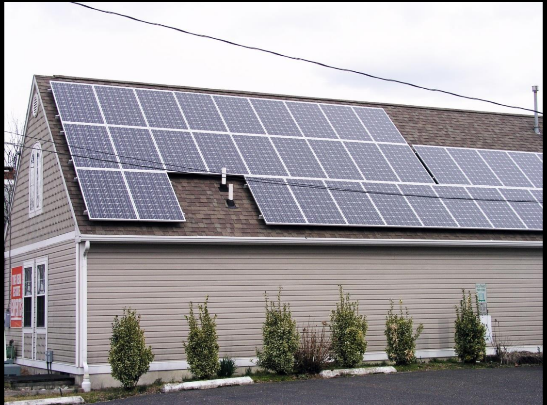
Above: Solar panels in Pemberton Township.
